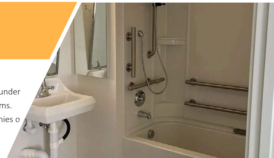
Bathrooms at Leigh Ave have medicine cabinets but limited storage options for larger items.
